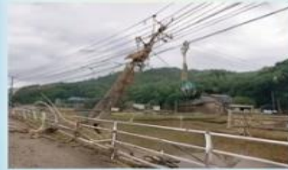
Damage in Mabi Town, Kurashiki City, Okayama Prefecture from July 2018 heavy rain
